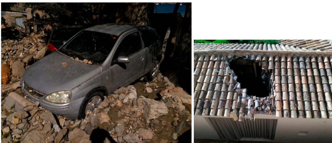
Fig. A2. Es Cubells (Ibiza), damages caused by the heavy rainfall event in August 2017. ©Emergency Service from the Balearic Islands.
