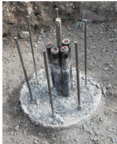
Figure 1. Example of a pile heat exchanger following pile trimming and prior to connection to the building base slab and the ground-source heat pump system. In this particular case the heat transfer pipes are centrally located and still retain their protective sleeves, which were used to avoid their damage during trimming.
