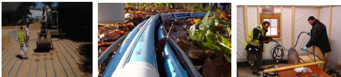
Figure 2. Deployment of one horizontal heat exchanger sector; HDPE pipe with its fiber along; fiber handling in the hut
