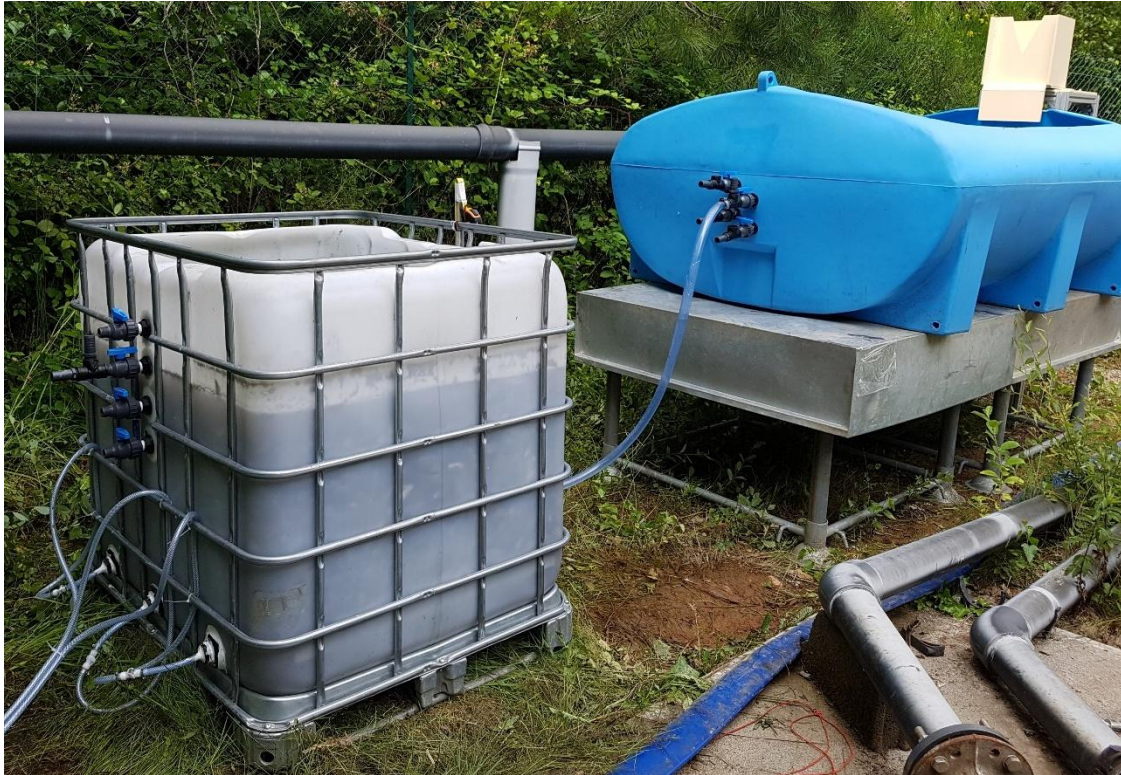
Figure 2 Picture of the pilot plant on site
