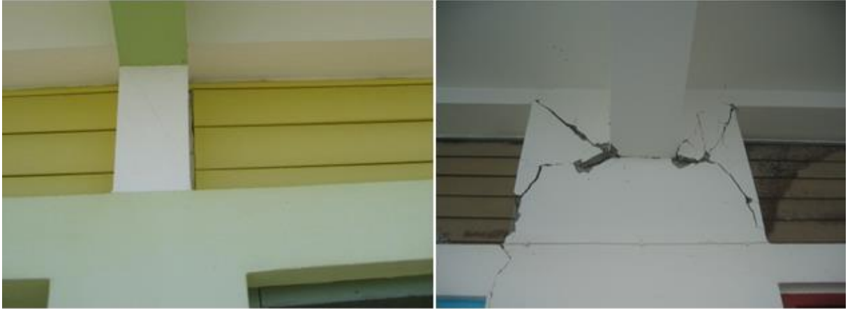
Figure 1: Diagonal cracks in the short columns
