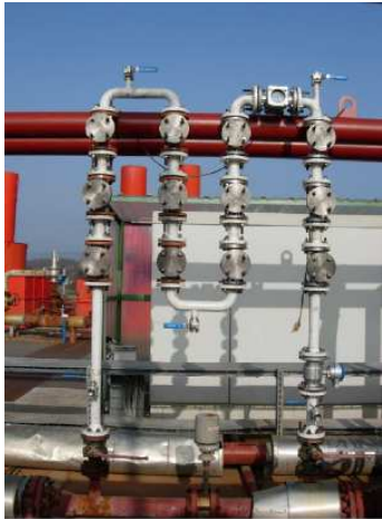
Figure 12: Corrosion and coating study with the High Temperature Skid installed on the Soultz plant (picture GEIE).
