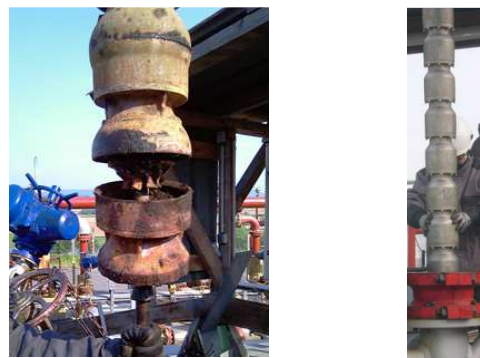
Figure 14: Status of the hydraulic part of the LSP pump after the pull operation of April 2011 (left) and picture of the new hydraulic LSP pump (right).
