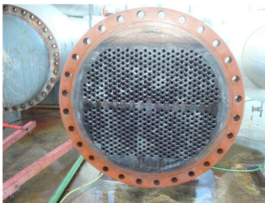
Figure 13: Black scaling observed within the heat exchanger during exploitation.
