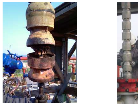
Figure 14: Status of the hydraulic part of the LSP pump after the pull operation of April 2011 (left) and picture of the new hydraulic LSP pump (right).
