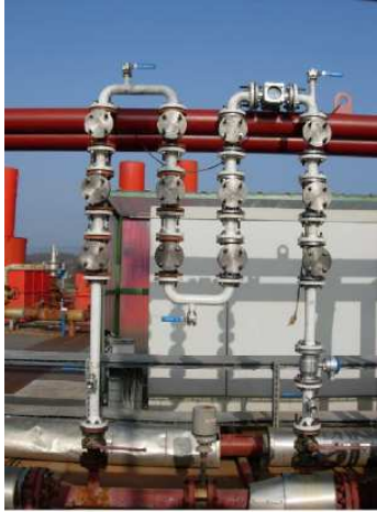
Figure 12: Corrosion and coating study with the High Temperature Skid installed on the Soutz plant (picture GEIE).
