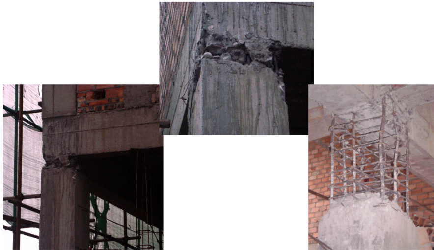
Figure 2 – Examples of damage to RC frame buildings. Photographs taken by S. Ghavamian in Dujiangyan following the 2008 Sichuan earthquake
