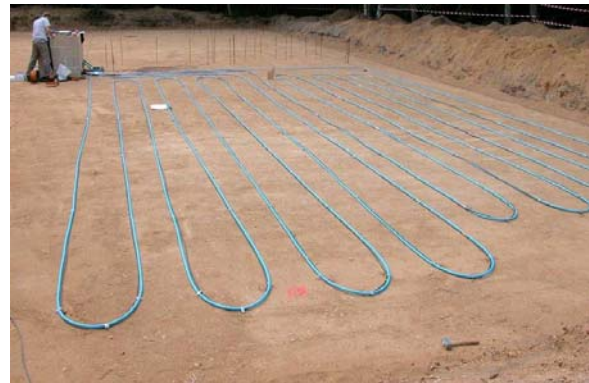
Figure 3: Equipment of one horizontal ground heat exchanger sector by its 2 fluid loops at 1 m depth
