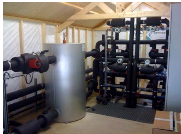
Figure 4: Thermodynamic machinery implemented in the hut
